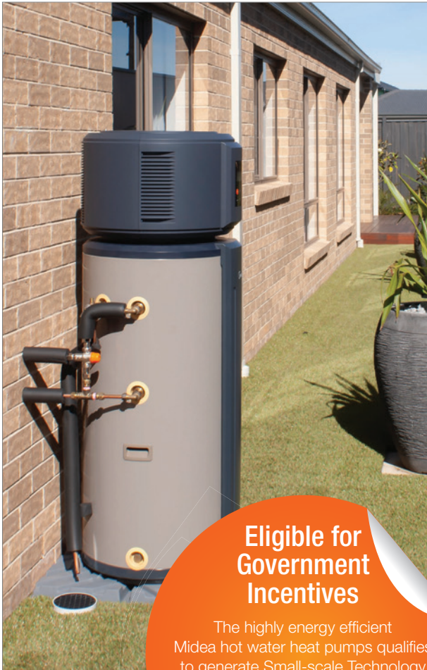
170L Installed Unit
